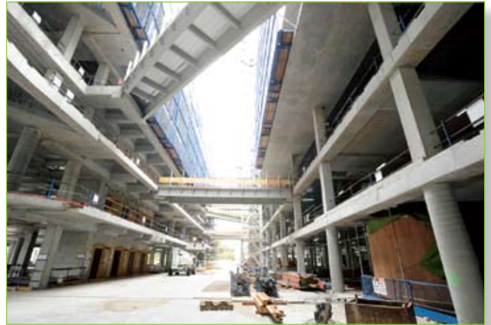
Pedestrian bridges connecting the west and east buildings are being constructed above 'the street'—the public walkway based on the concept of a Victorian town's main street.
