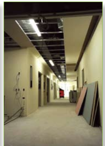
Right: Inside the inpatient building, sheeting has been fitted to walls, services are being installed and ground services prepared for the installation of flooring.
