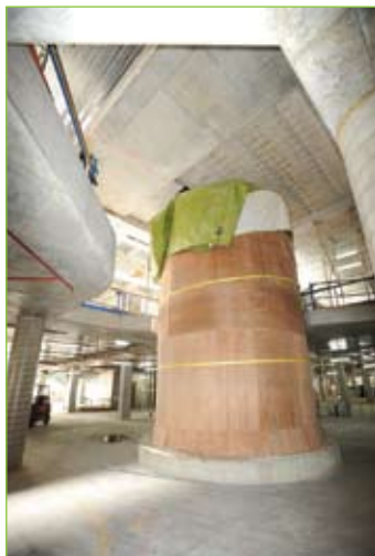
Left: The aquarium, which will be a wonderful visual highlight of 'the street' and Emergency, is concealed in protective wrapping. It needed to be placed on site so the surrounding building structure could be completed.
